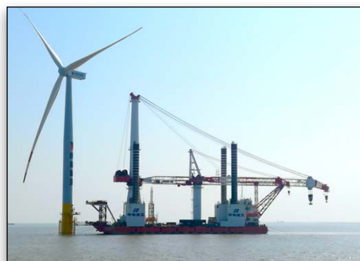
The project team used Bentley's OpenWindPower to optimize the construction and operation of this large wind power project.
